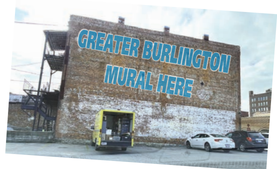
Watch the progress wall of Jennison Building (Drake overflow parking lot), 410 N Main Street
